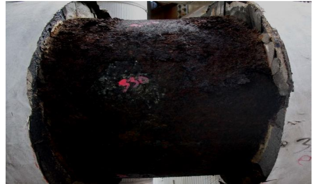
Figure 12: CUI becomes a significant issue when insulation plugs are removed but not replaced and resealed again (PetroChem Inspection Services Inc, used with permission)
