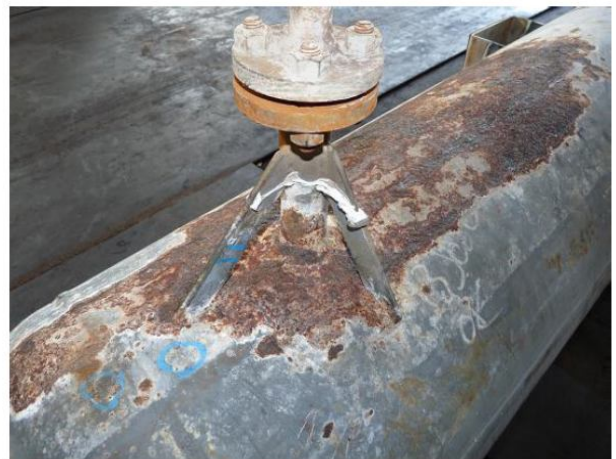
Figure 3: CUI as induced on inorganic zinc coating after working for 8 years in a coastal industrial atmosphere: Note the steam inlet nozzle and the effect of water ingress around it. © National Corrosion Association (NACE) 10
